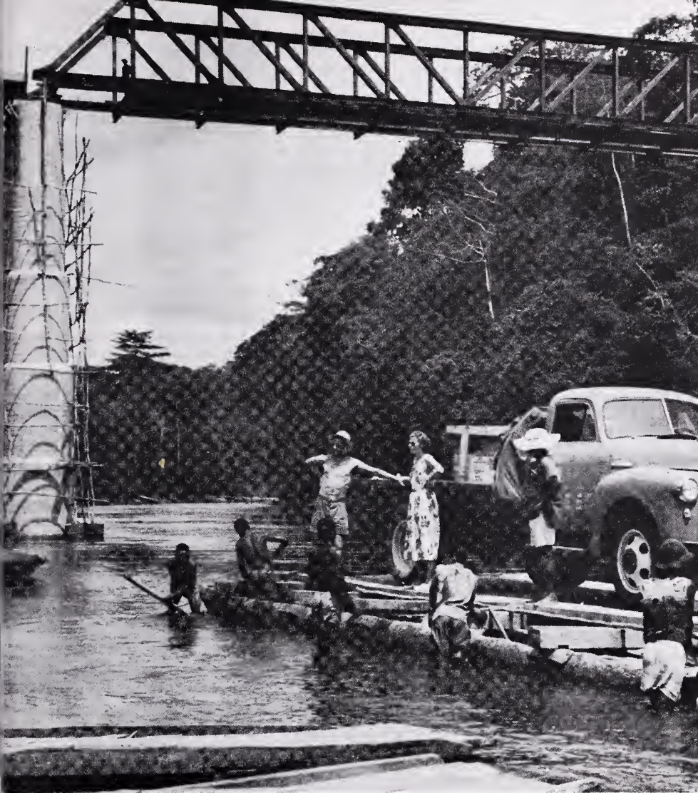
New roads and bridges are opening up remote and rugged areas of the British Cameroons. This bridge, in Bamenda, will replace a primitive ferry in the Trust Territory. Visiting Missions have stressed the formidable obstacles to roadmaking in the territory which, in 1953, had something over 1,500 miles of motorable roads.
